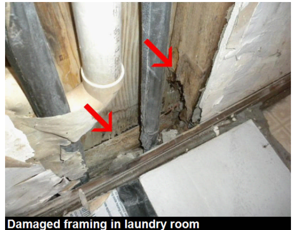
Damaged framing in laundry room
