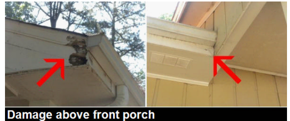
Damage above front porch
