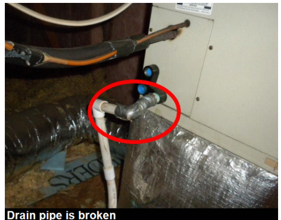
Drain pipe is broken
