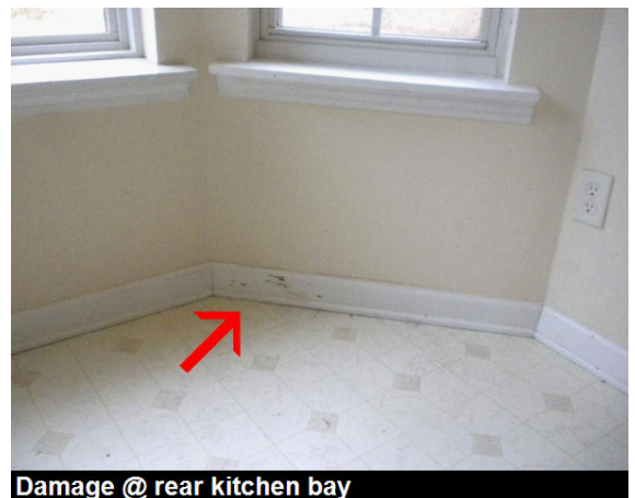
Damage @ rear kitchen bay
