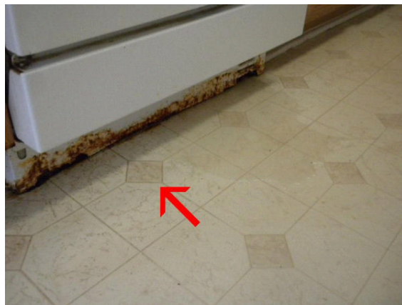
Dishwasher is leaking
