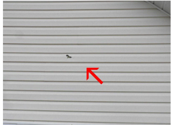
Damaged siding above the garage
