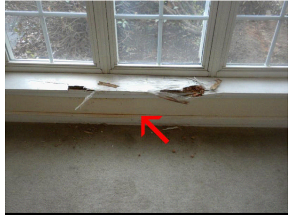
Damage @ dining room window
