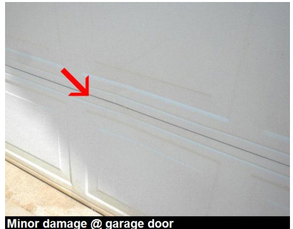
Minor damage @ garage door
