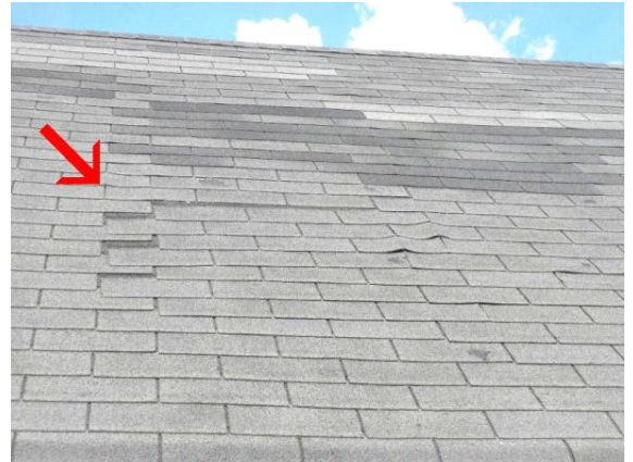
Loose shingles @ right side of the house
