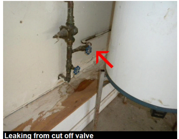
Leaking from cut off valve
