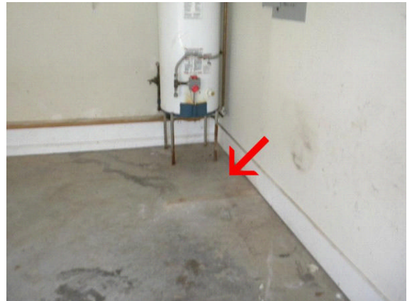
Install barrier in front of water heater
