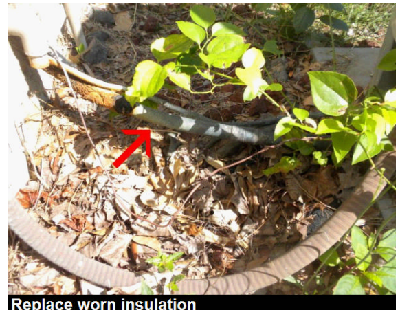
Replace worn insulation
