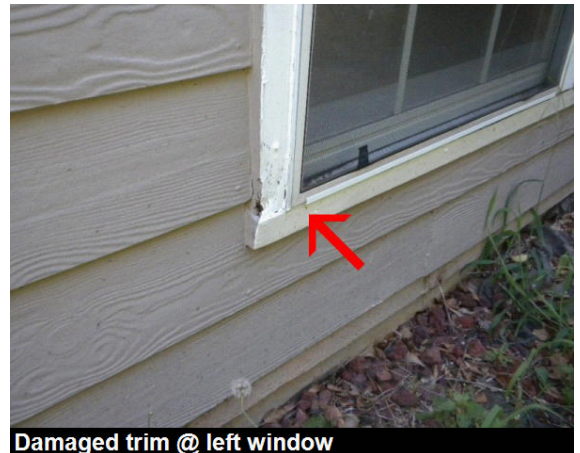
Damaged trim @ left window
