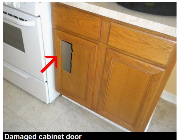
Damaged cabinet door
