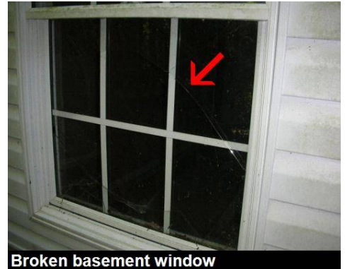
Broken basement window
