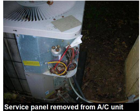
Service panel removed from A/C unit
