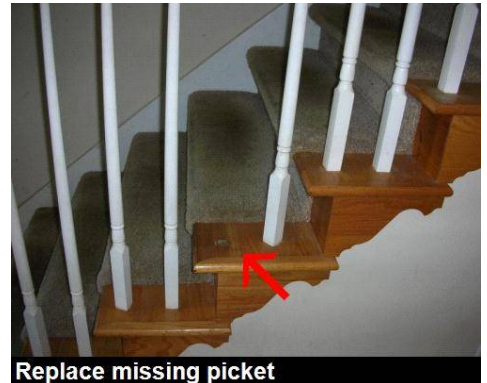
Replace missing picket
