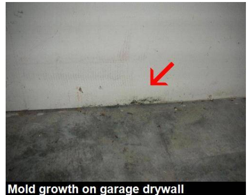
Mold growth on garage drywall
