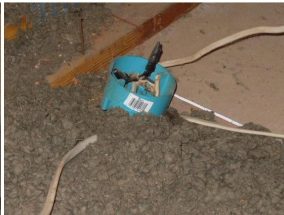
Open junction box
