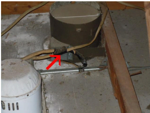
Open wire splices
