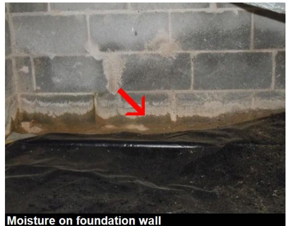
Moisture on foundation wall
