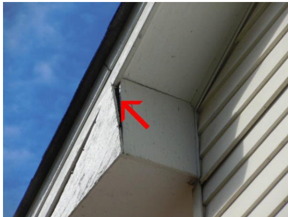
Fascia pulling loose
