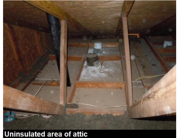
Uninsulated area of attic
