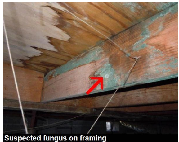
Suspected fungus on framing
