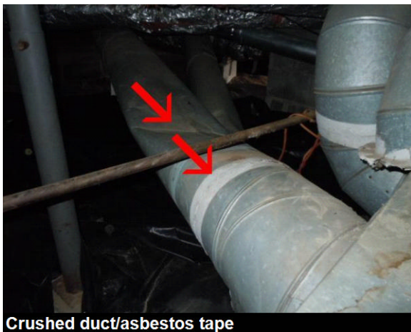
Crushed duct/asbestos tape
