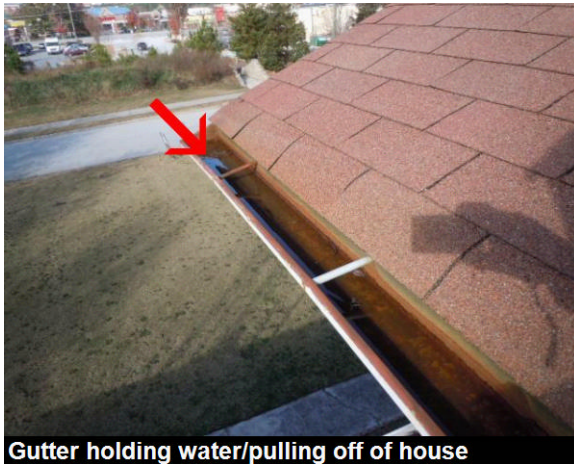
Gutter holding water/pulling off of house
