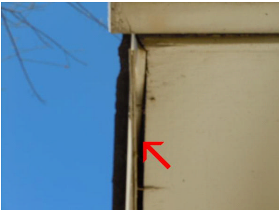
Fascia pulling loose
