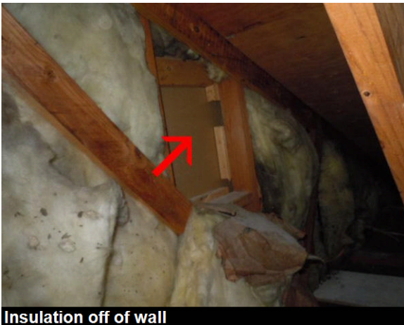
Insulation off of wall
