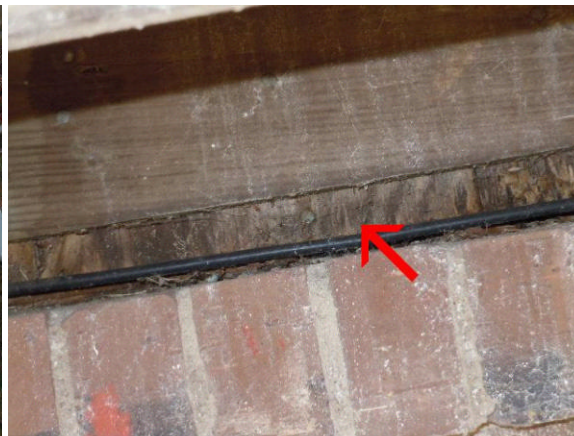
Decayed siding under stoop
